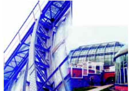
Main tropical greenhouse in the Botanical Garden with a section of the old steel construction
